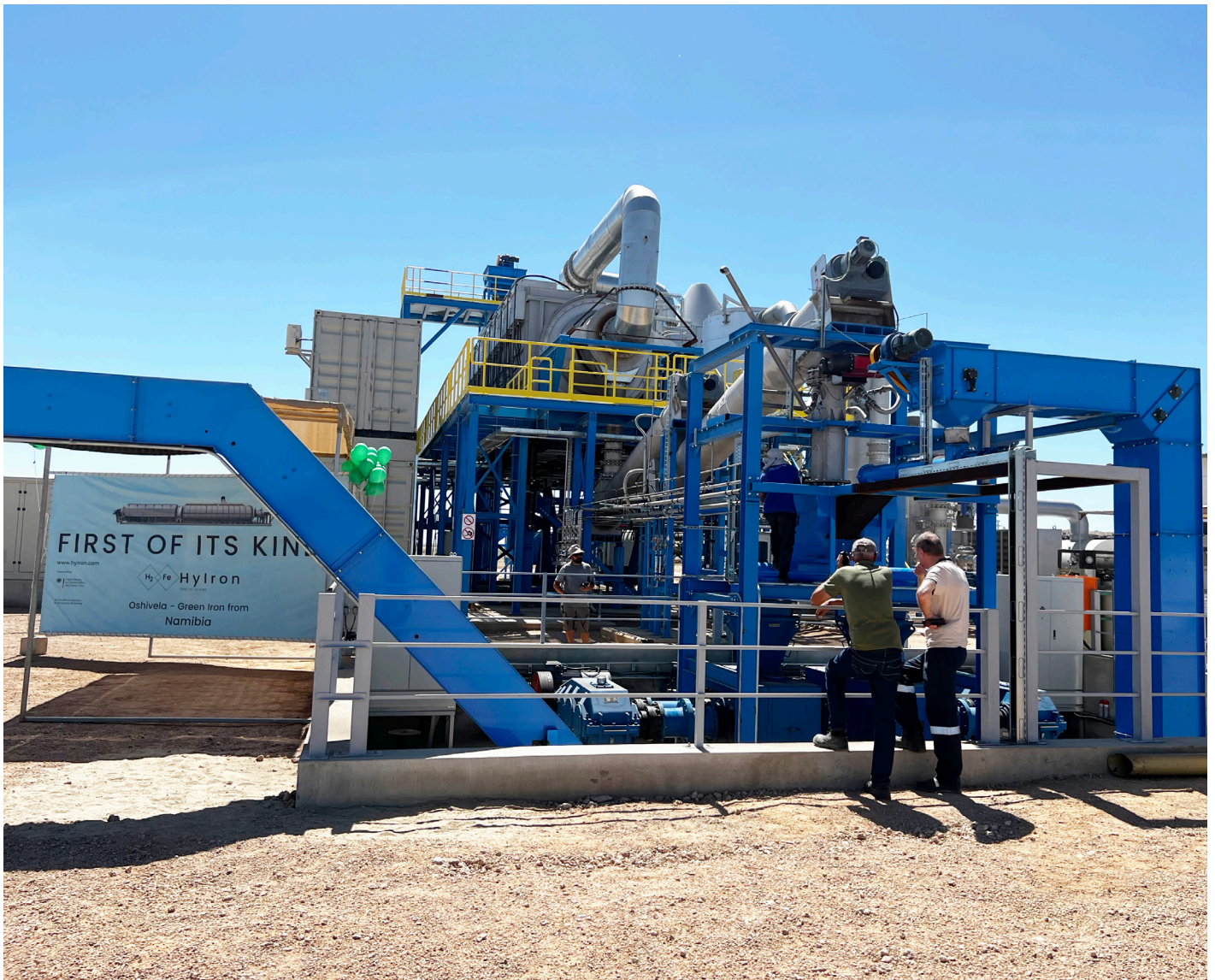
The plant at HyIron's Oshivela green iron facility in the Erongo Region. (Source: NGH2P)
